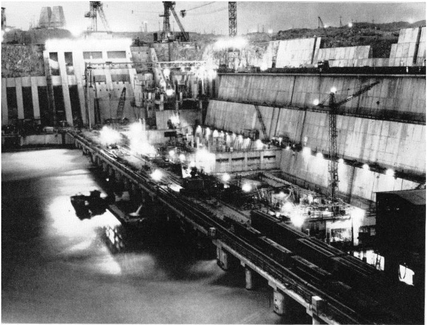
Night view of second stage work on the Aswan Dam Power Station, part of the massive structure across which the Tropospheric Scatter System will fire [Reproduced by courtesy of the United Arab Republic]
