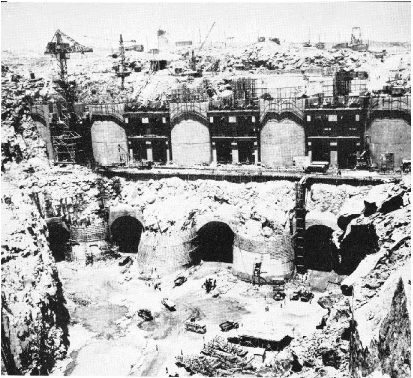
Four of the six colossal hydraulic tunnels that were dug out of the rock. Above can be seen the foundation of the hydro-electric power station [Camera Press]
