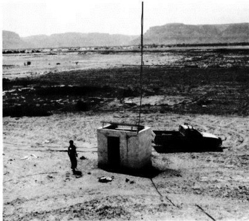
One of the two repeater stations. The solar panel can be seen on top of the building
